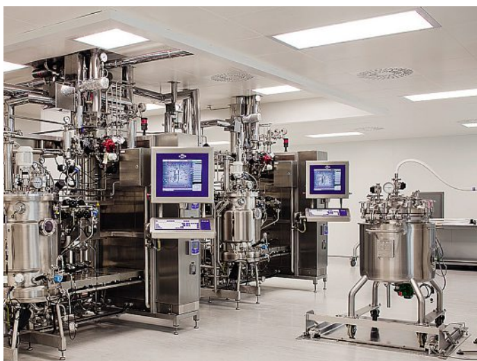
Upstream processing suite at the National Institute for Bioprocessing Research & Training (NIBRT) in Dublin, showing two completely controlled 150-litre perfusion bioreactors (left of image) and harvest vessel (on right of image). (Copyright NIBRT)
